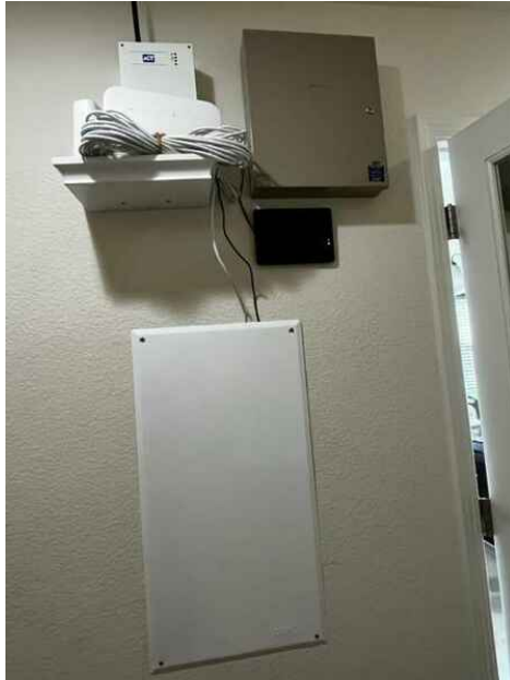
Alarm System Panel located in Primary Bedroom closet.
