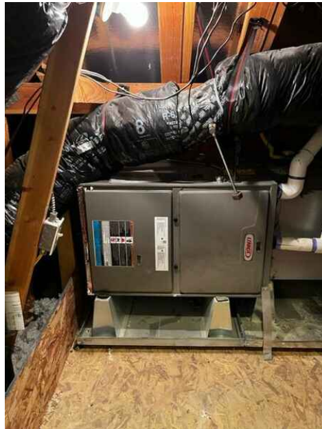
Furnace located in Loft Room closet.
